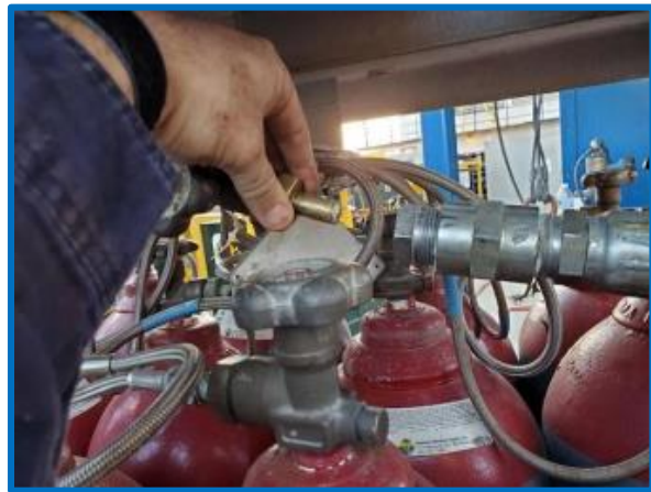
Incident 2: Failed Hose Connection on Bottle Rack.
