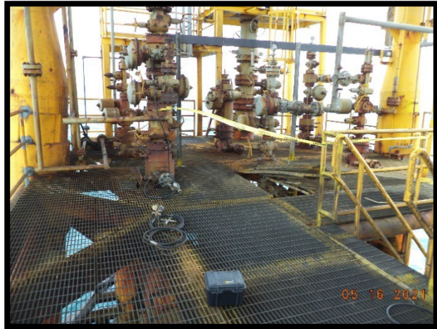
Figure 5– Photograph of Upper Deck with Pressure Regulator, High Pressure Hose, and Black Case Laying on Deck
