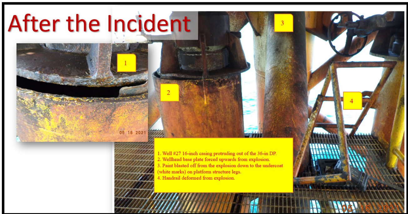
Figure 8 – Photograph of Incident Scene Showing Effect of Explosion
