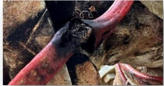
Fig 3 - Damaged insulation on heat trace cable routed along the top of the inlet flange.
