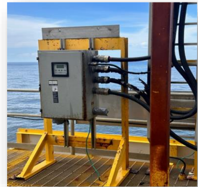
Fig. 4 - Junction Box (400 Automatic Transfer Switch).
