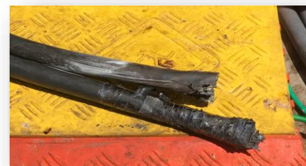
Fig.2 - #2 phase cable melted off lug connection.
