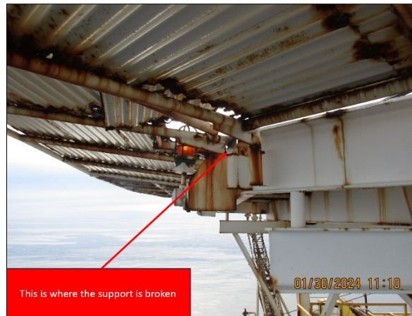
Figure 2. Damaged skirting substructure.
