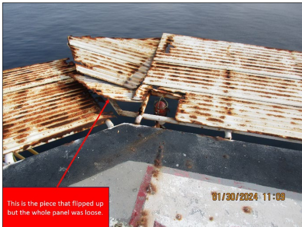
Figure 1. Damaged helideck skirting.
