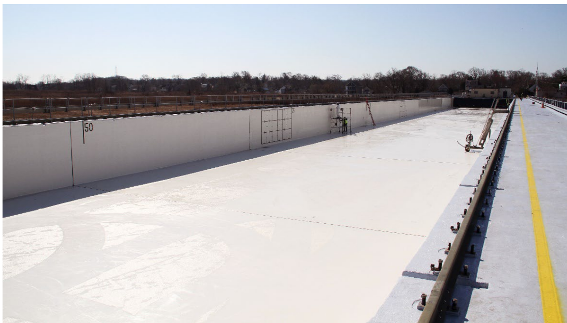
Figure 7. View of empty tank showing fresh paint, concrete repair, and new sealants prior to it being refilled with Sandy Hook Bay seawater in a three-day operation. (Photo from Mike Brennan, BSEE)
