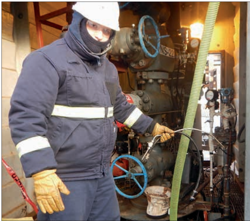
Soon after summer ends, BSEE's Alaska inspectors need to shield themselves from the elements. Because oil and gas production does not stop when the weather turns cold, BSEE's inspectors still need to visit Alaska's artificial Northstar Island, which lies in state waters, but has wells that extend to the federal OCS.
