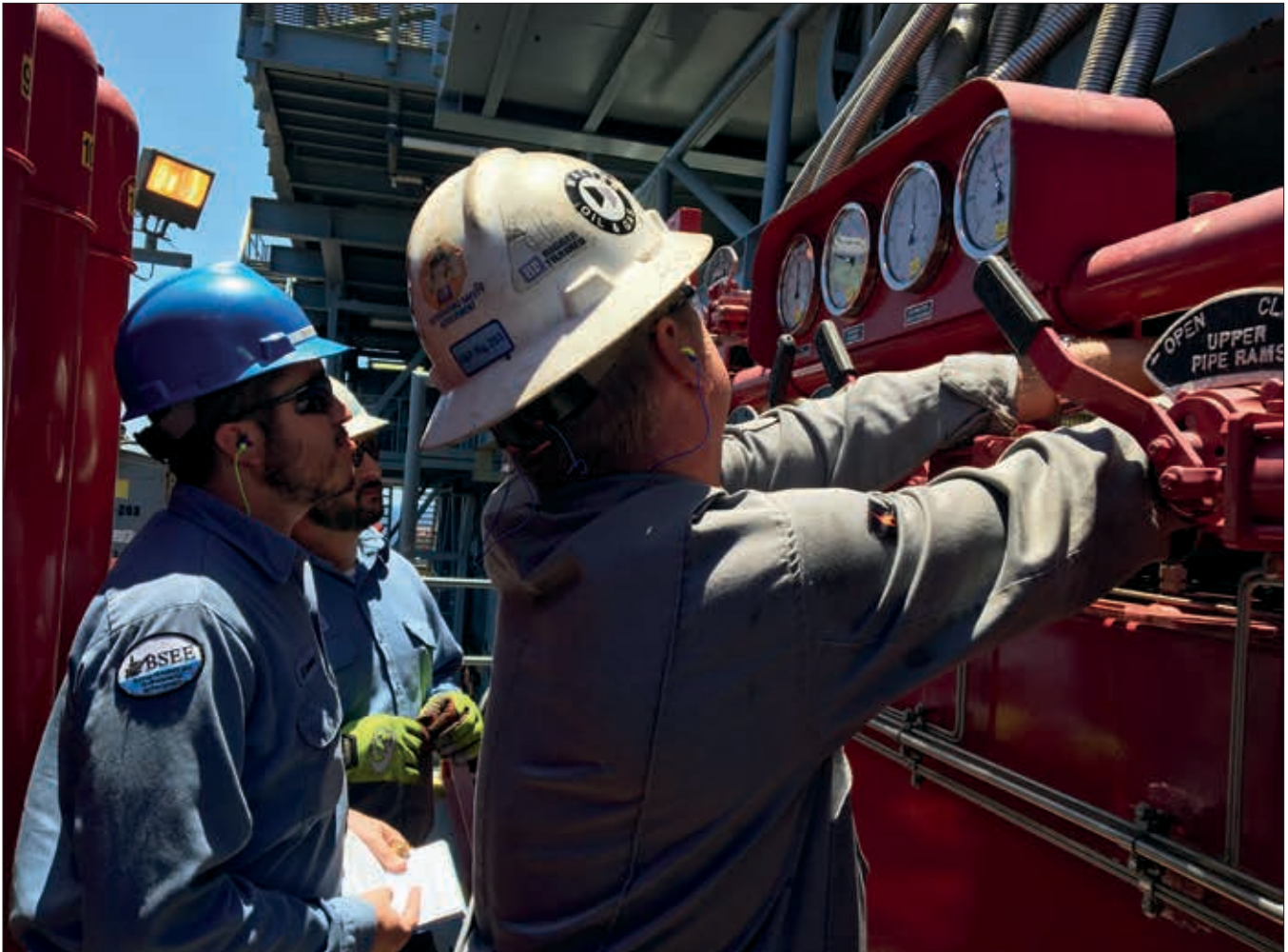
Inspectors from BSEE's New Orleans District Well Operations Unit observe the company's tool pusher as he conducts a successful test of the facility's accumulator.
