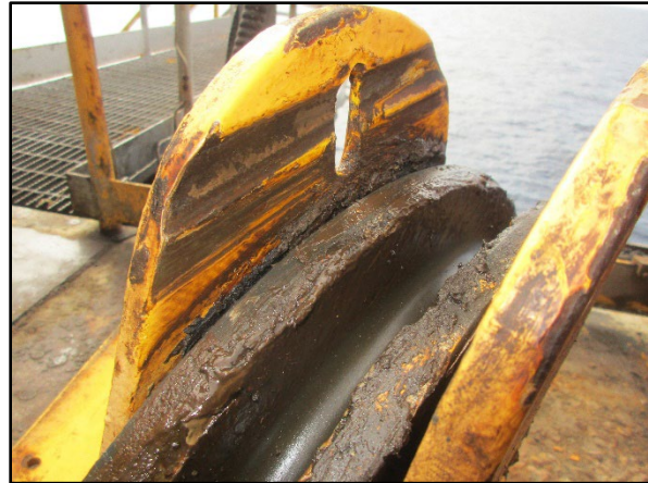
Inside abraded main line carrier sheave side plate that is missing rope guard.
