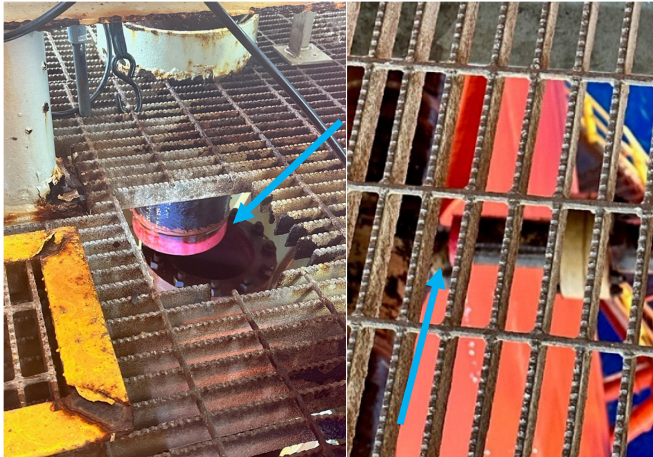
Figure 1: FRP pipes separated from flanges.
