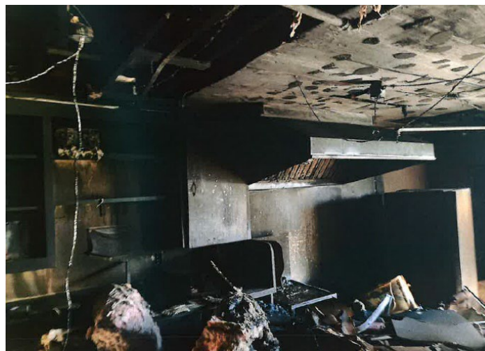
Figure: Fire spread to the living quarters following the removal of the heliport substructural frame using cutting torches.
