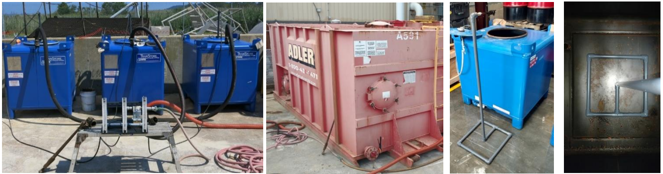
Figure 5 – Weathering Totes, Bulk Storage Tank, and Sparger Outside and Inside Tote
