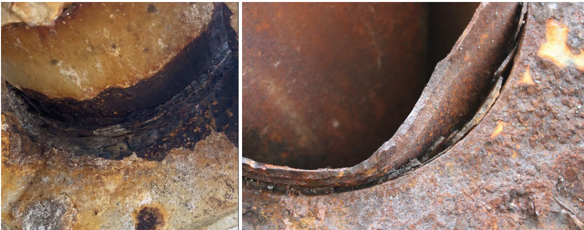
Figure 10: 10-3/4-inch Casing in Rocket Launcher from Top (Left) and Bottom (Right)
