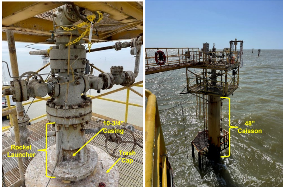
Figure 7: Annotated Elements of the Wellhead and Platform (Right Photo Taken from the L/B Swordfish)
