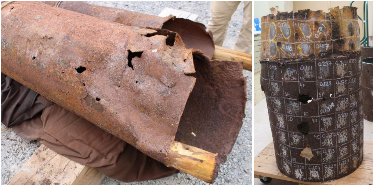
Figure 11: Corroded 20-inch Structural Casing After Recovery (Left) and After Cleaning for Thickness Measurements (Right)
