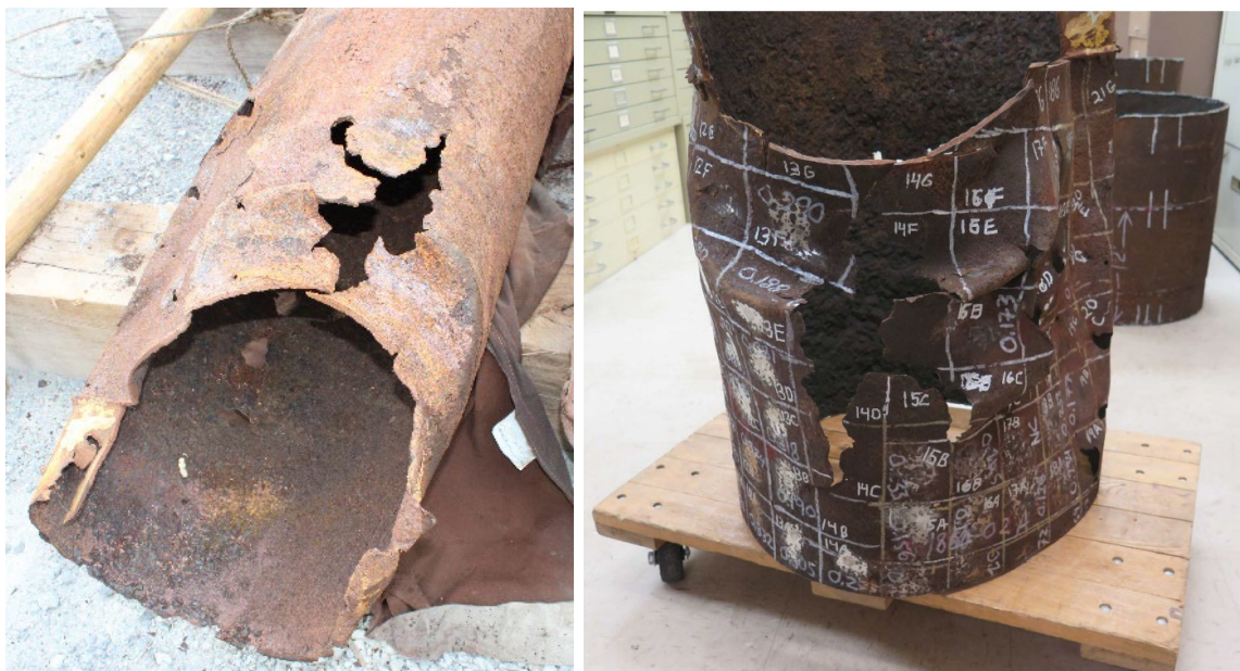
Figure 13: Buckled 20-inch Structural Casing After Recovery (Left) and After Cleaning for Thickness Measurements (Right)
