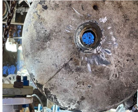
Figure 2. Nozzle removed from top of vessel.
