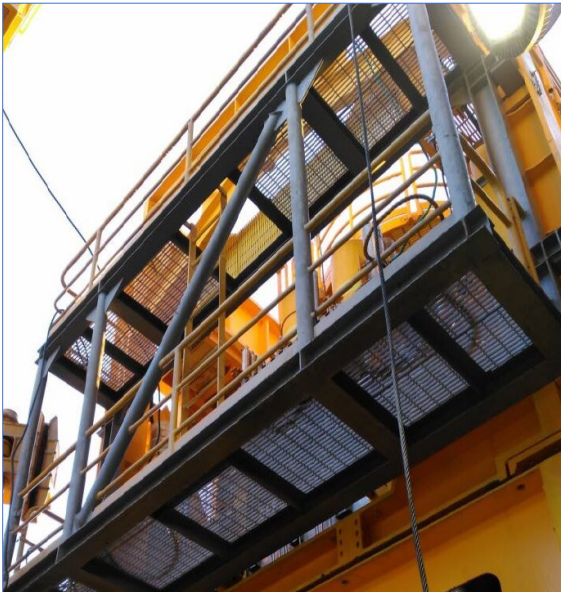
Figure 1. Blowout preventer work platform.
