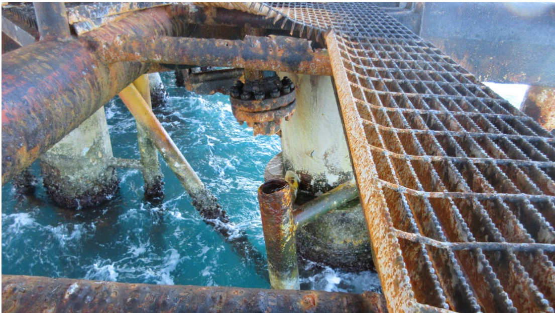
Figure 1. 8-inch bi-directional gas pipeline failure and damaged grating.
