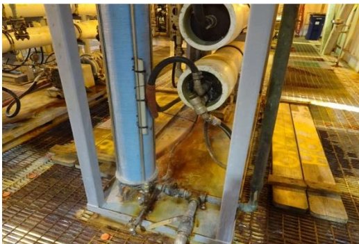
Figure 1: Faulty grating covered in scaffold boards (right).
