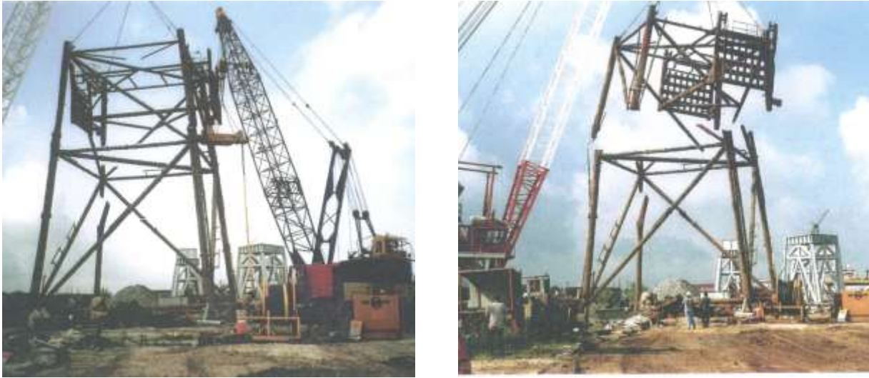
Figure 6-25. Power Shear Cutting Platform Jacket (Photo courtesy of Prime Marine Services, Inc.)
