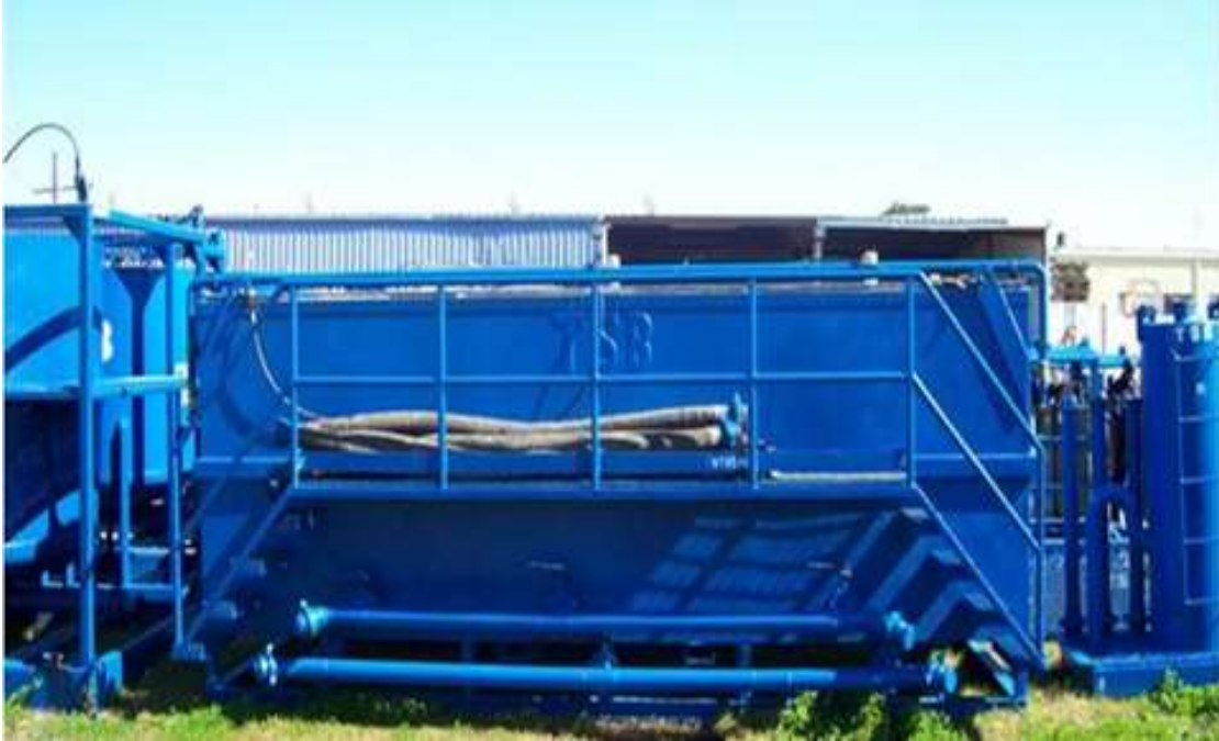
Figure 6-4. Rigless P&A Return Tank
