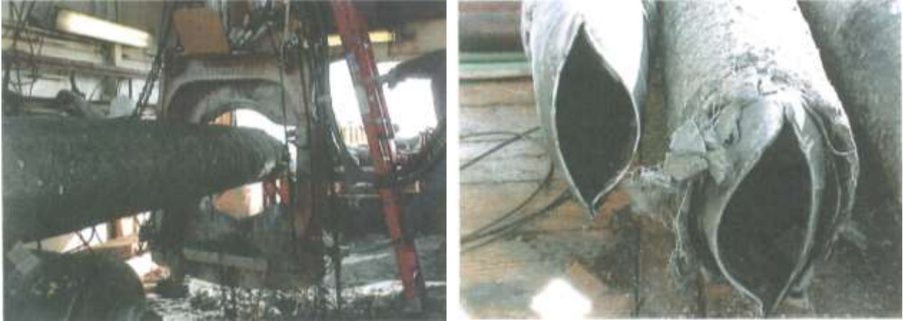
Figure 6-23. Pipeline Cut with Power Shear (Photo courtesy of Prime Marine Services, Inc.)
