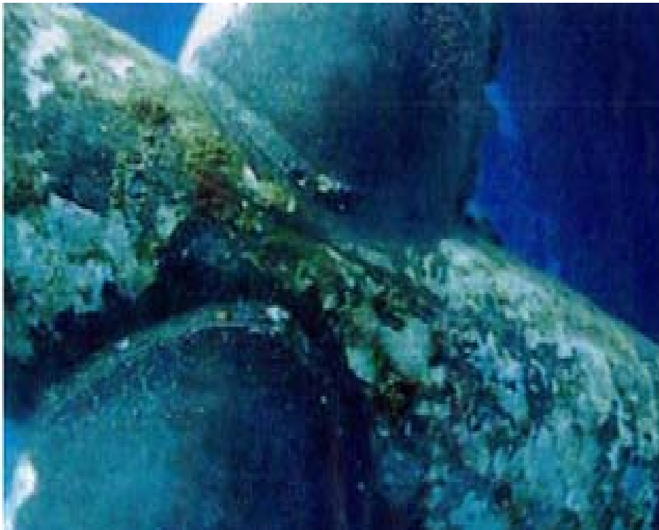
Figure 1.4 Damaged X-joint of a Platform
