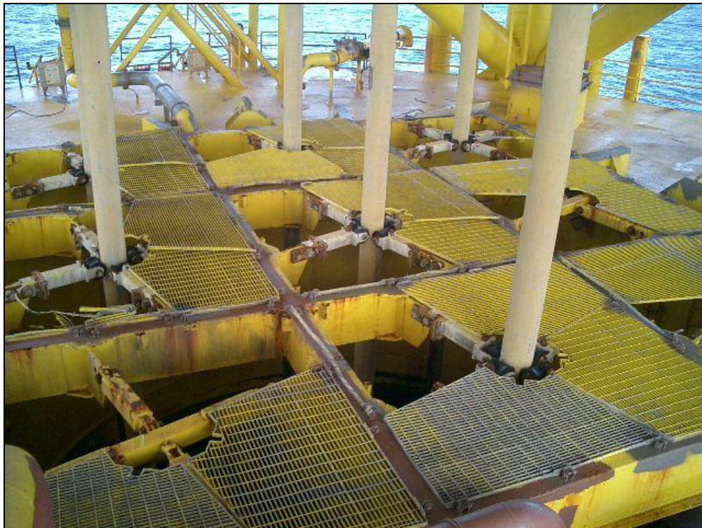
Figure 6.3 Missing Grating around Risers in Moon Pool
