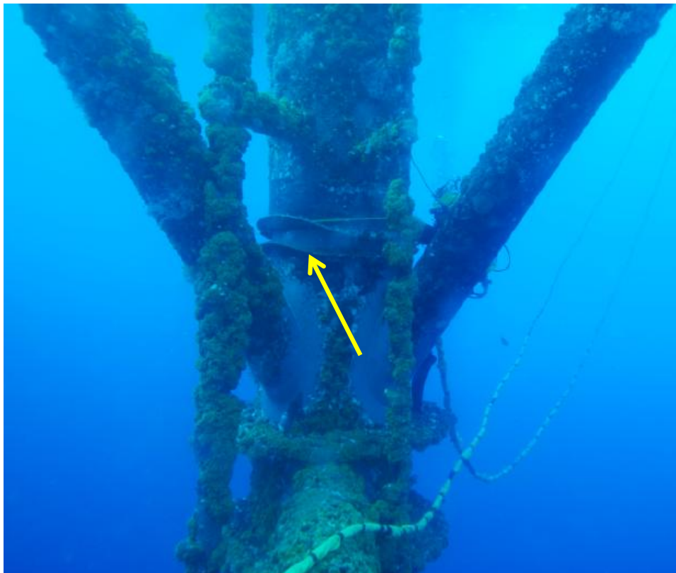
Figure 5.26 Pancake Leg Damage – Final Damage Configuration (VR 1)
