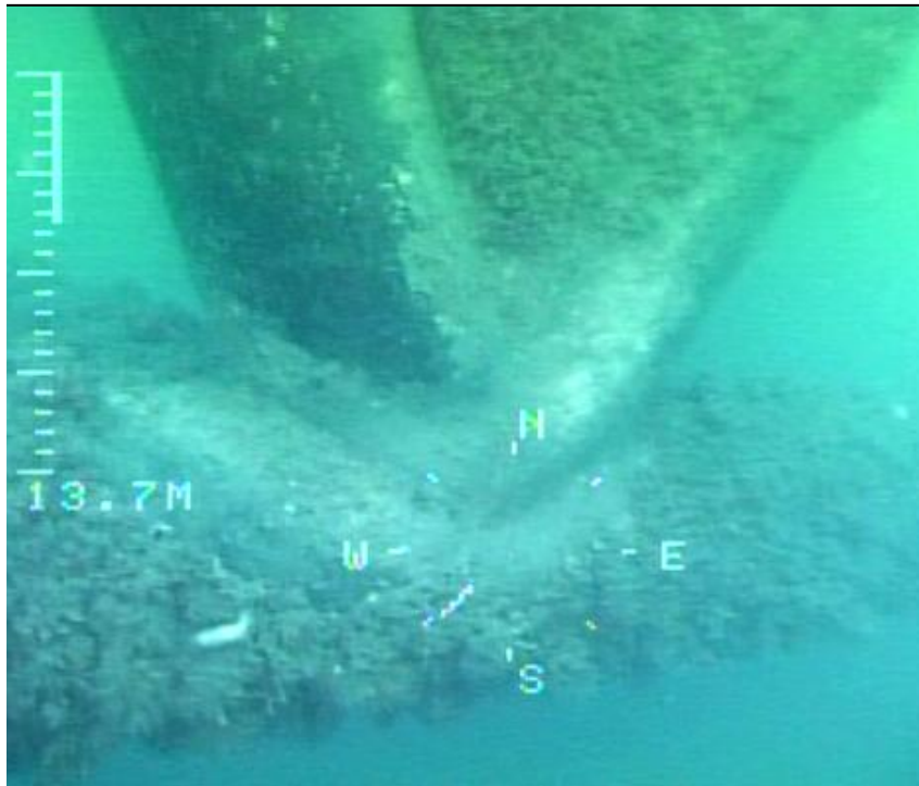
Figure 6.7 Damaged K-brace Node (Note missing marine growth indicating high stress region)
