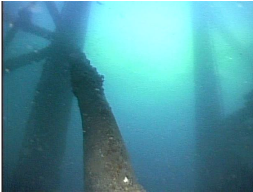
Figure 6.6 Out of Plane Bowing of Vertical Diagonal Brace (Note missing marine growth indicating high stress region)
