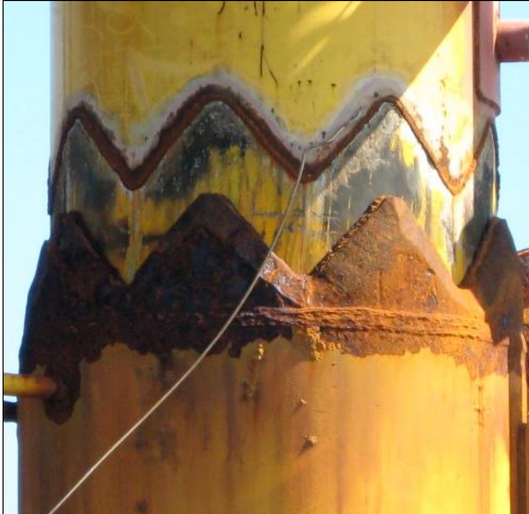
Figure 6.12 Crown Shim Failure due to Inadequate Welding
