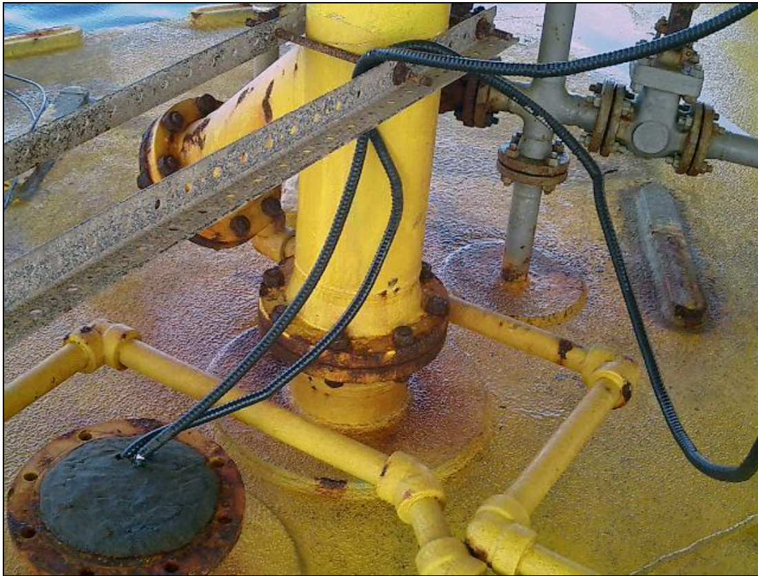
Figure 6.4 Cable Tray Damage Top of hull
