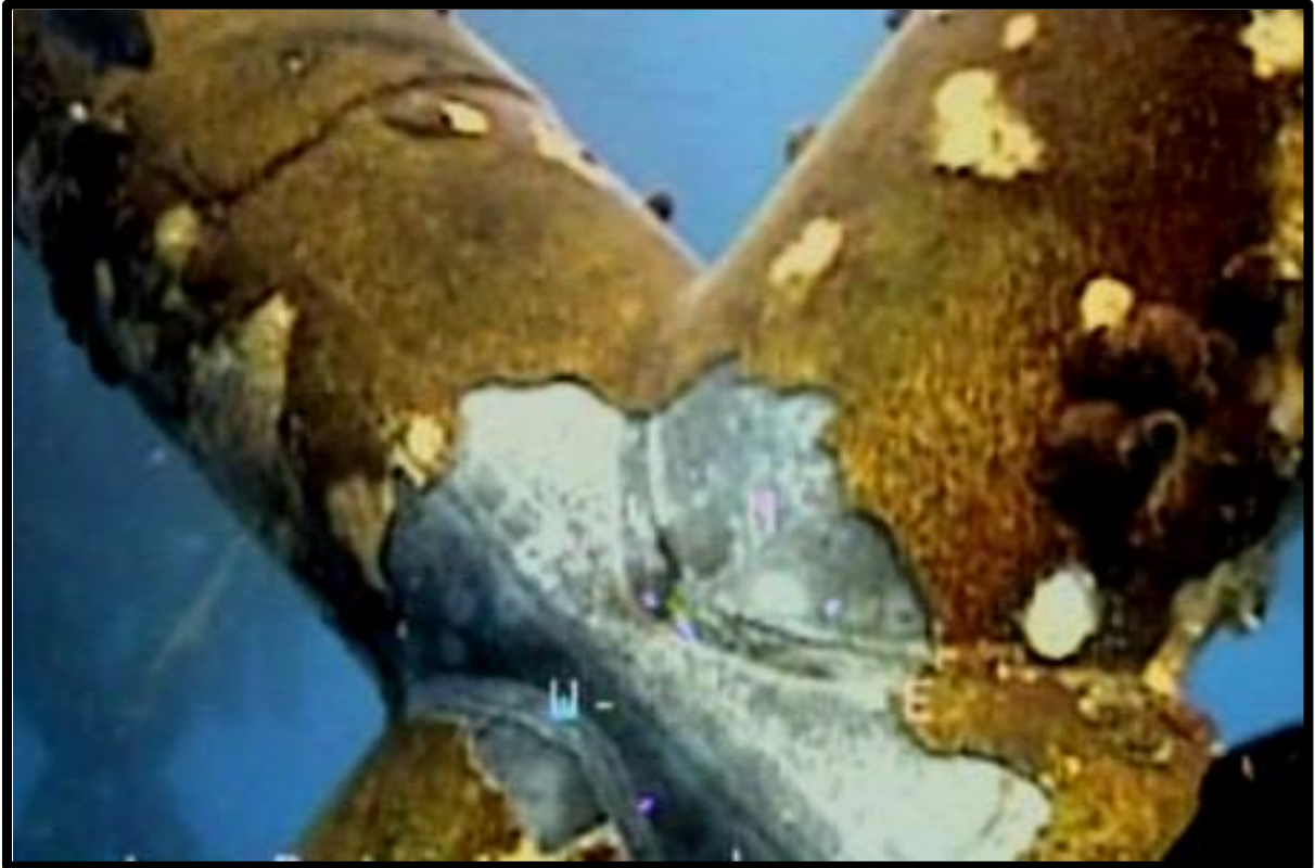
Figure 6.8 Crushed X-brace node (Note missing marine growth indicating high stress region)
