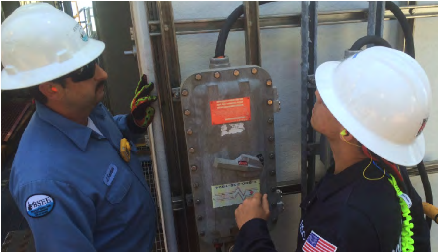
A Coast Guard inspector (right) and his BSEE counterpart examine a cable connection on an offshore oil and gas platform.
