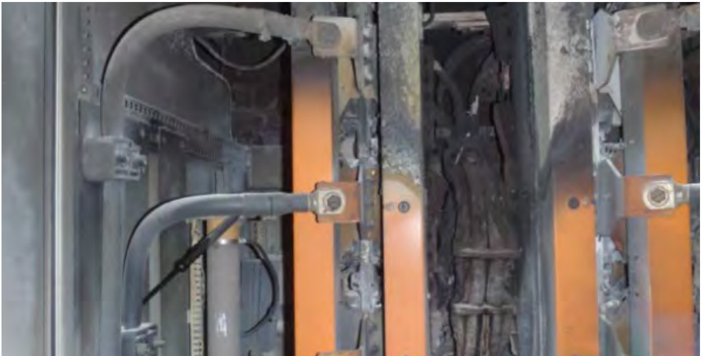
The charred component of this thruster reveals evidence of a fire. Working jointly, the Coast Guard and BSEE helped make sure that the drillship's maintenance, testing and inspection program addressed the underlying cause of this second fire that was tied to the same component.
